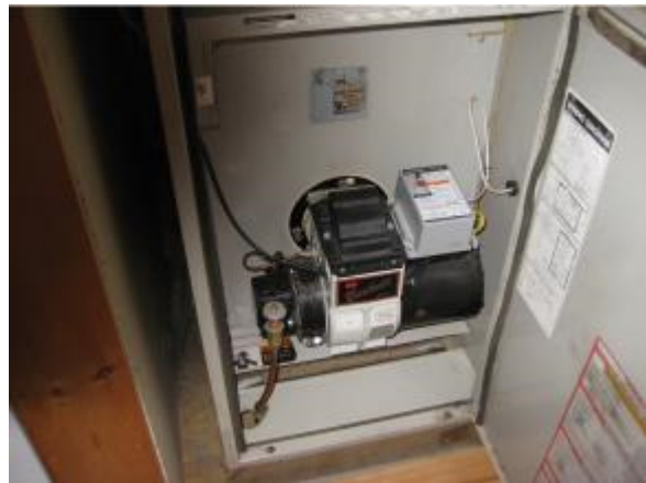
replaced? Hot Air Furnace
