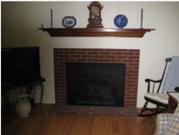
Wood, now Propane, Fireplace
