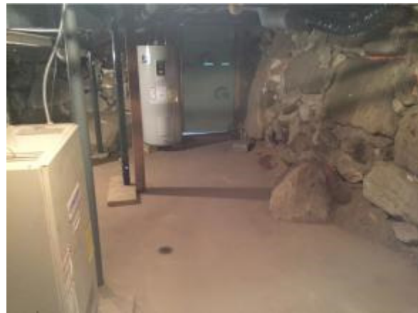
New HWH & Oil Tank
